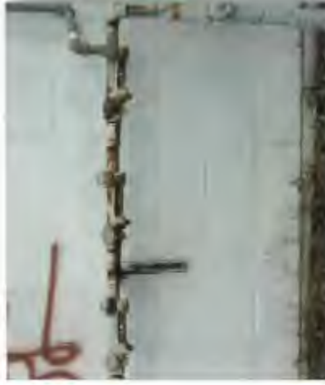
Meters Removed - Live Gas??
