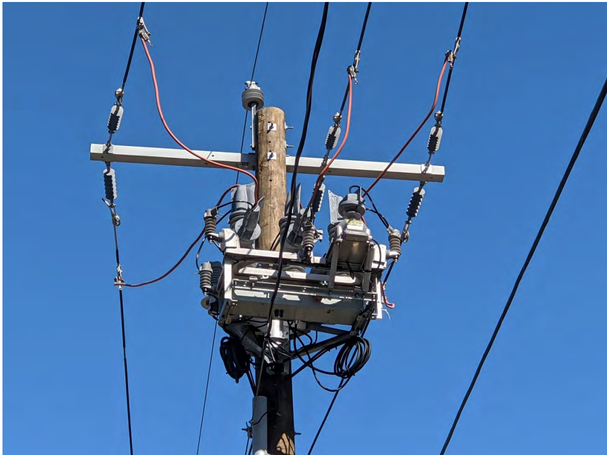
Figure 7. Eversource Overhead Recloser
