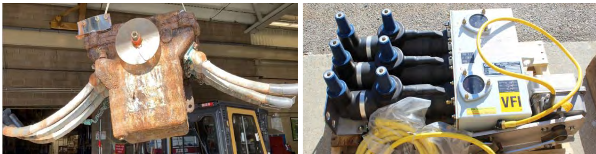
Figure 6. Old Oil-Filled Switches (Left) and New VFI Switches (Right)
