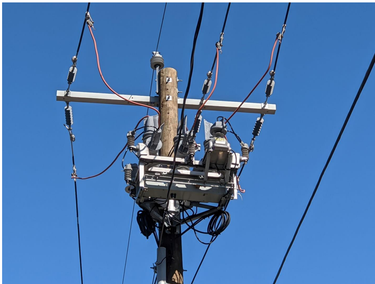
Figure 8. Eversource Overhead Recloser
