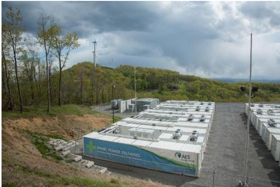
Figure 1-15: AES Laurel Mountain Energy Storage Project in West Virginia
