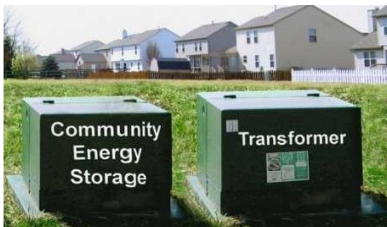
Figure 2-23: Community energy storage as utility infrastructure 91
