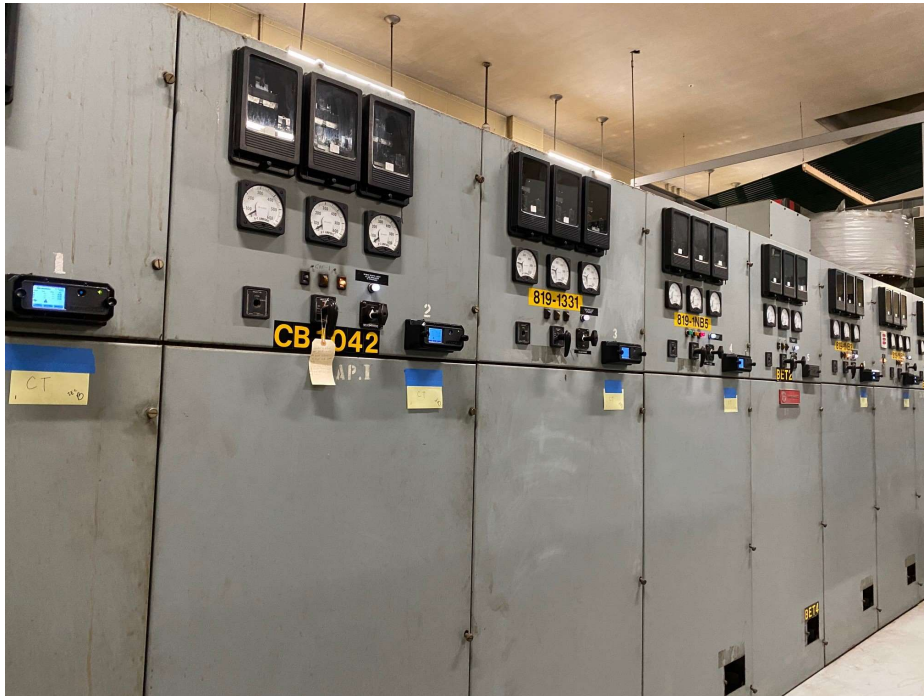
Switchgear Lineup with SMART Block Devices Installed
