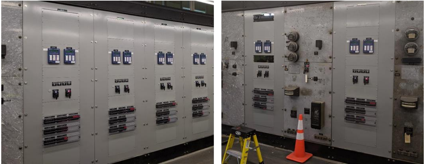
Figure 16: Depiction of newly installed relays (picture, left) and a combination of new and existing relays (picture, right). The existing relays in this 4kV substation were built into marble panels.
