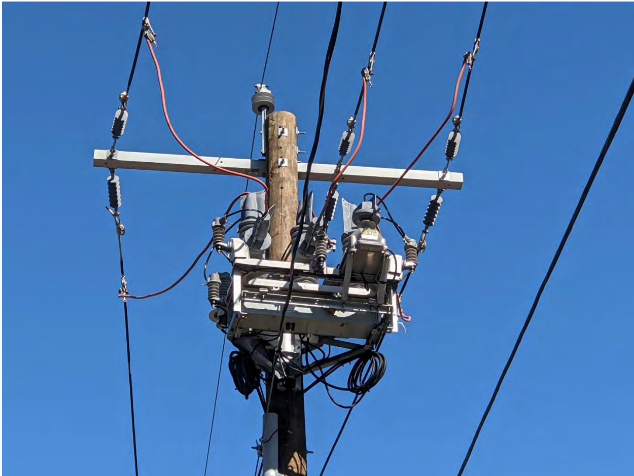
Figure 8. Eversource Overhead Recloser
