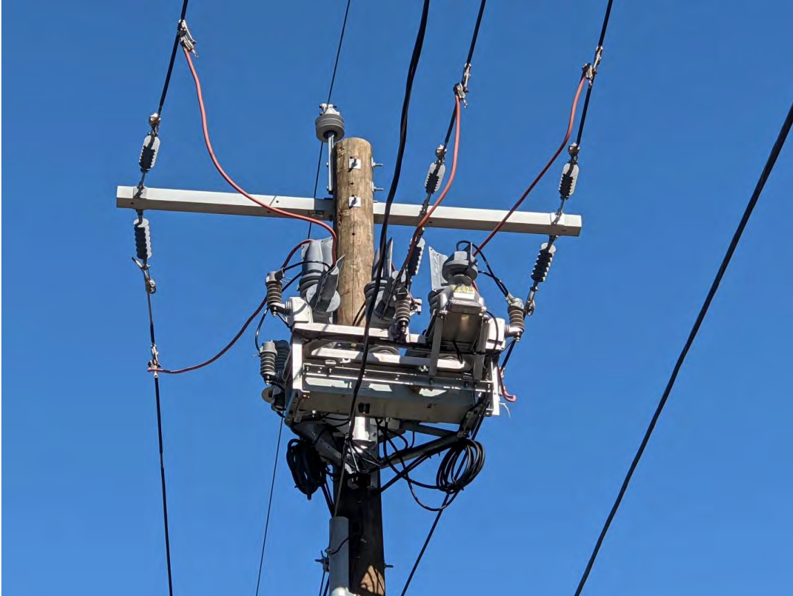
Figure 8. Eversource Overhead Recloser
