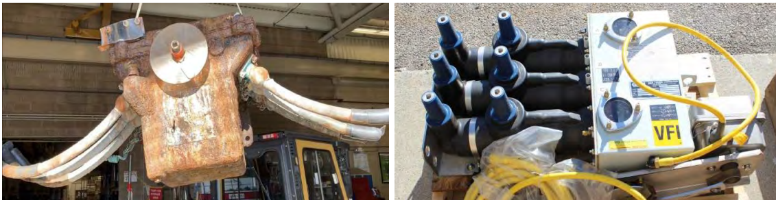
Figure 7. Old Oil-Filled Switches (Left) and New VFI Switches (Right)
