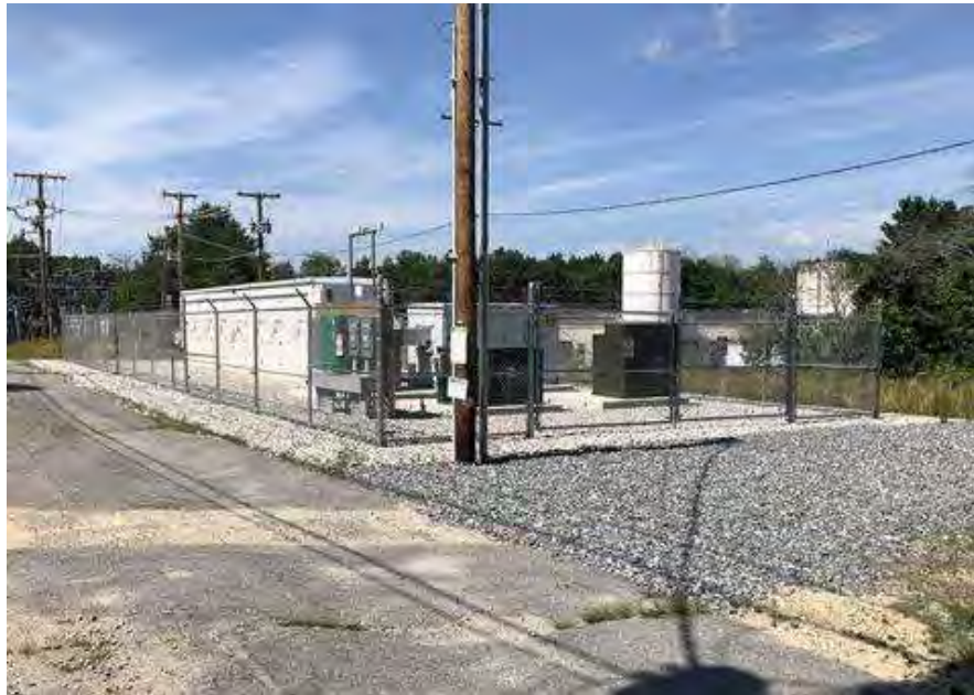
Figure 23: Energy Storage System at the Townsend Substation (Source: Unitil)
