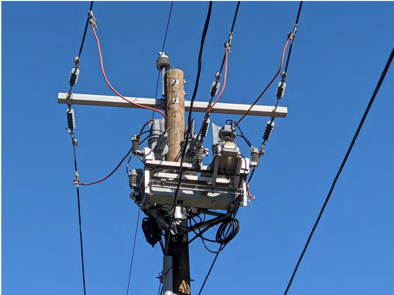
Figure 11. Eversource Overhead Recloser
