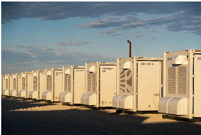
Crossett 200 MW, 200 MWh
