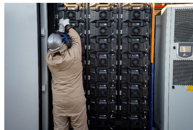
Swoose I 9.9 MW, 19.8 MWh
